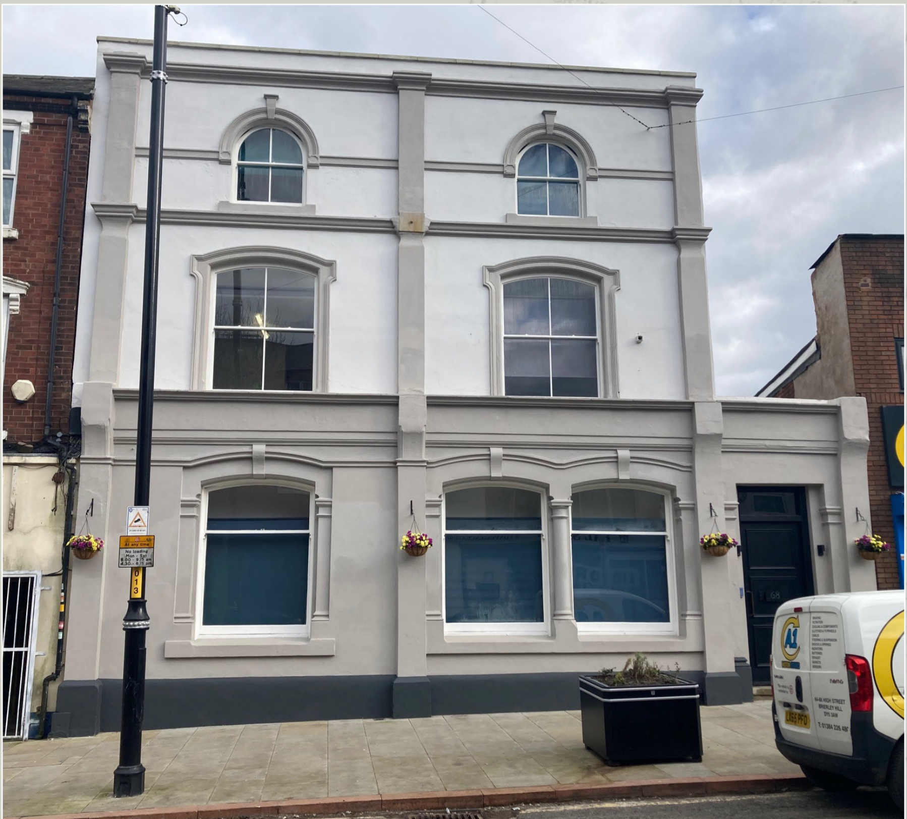
68 High Street in 2024 after it had been repaired thanks to funding through the Brierley Hill High Street Heritage Action Zone.
